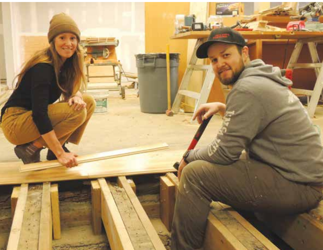
▲ Kara and Kyle Hellyer worked with contractors to rebuild the store. PHOTO BY CHRIS HAMILTON.
